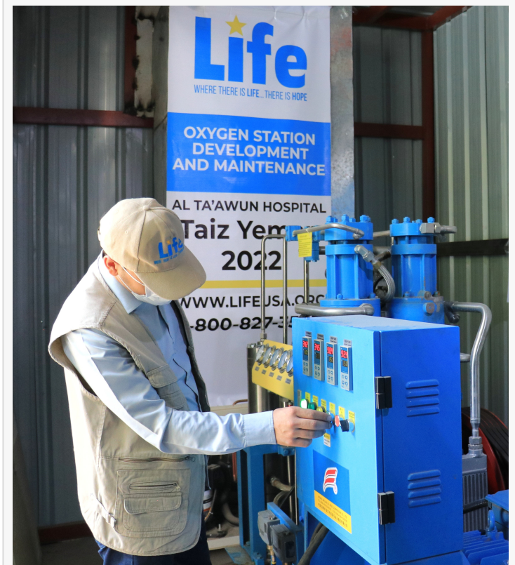
Yemen Oxygen Tank Station in Al-Ta'awun Hospital, Yemen
